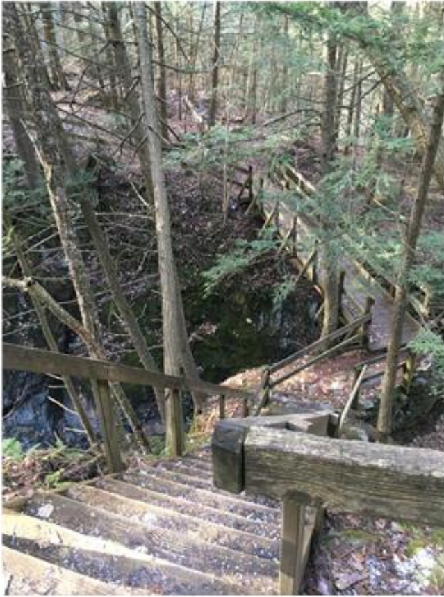
Figure 4. Original wooden staircase leading to footbridge over chasm for viewing Burnham Falls. Due to deteriorating conditions and safety concerns, this staircase was dismantled in the fall of 2019, and the bridge trail was closed until further notice.
